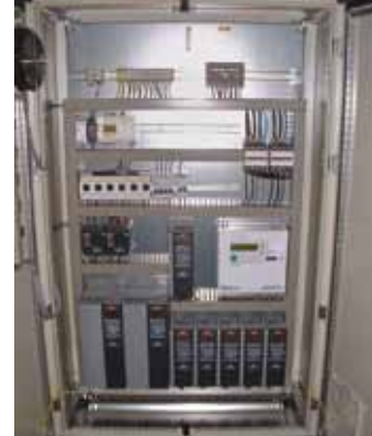
Fireman's Override Switch
